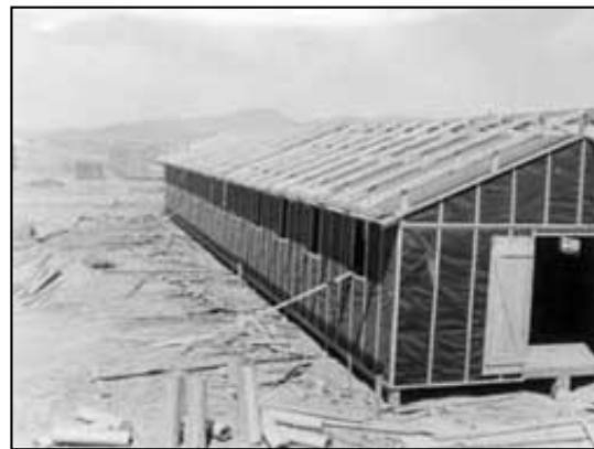
Figure 10.5. Construction underway at Poston I. (Fred Clark photograph, Bancroft Library, University of California, Berkeley)
